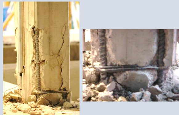
Tensile lap-splice failure of the column at the bottom
